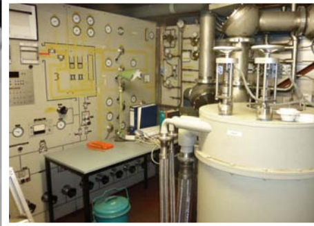
This was the control room of the cold source.
