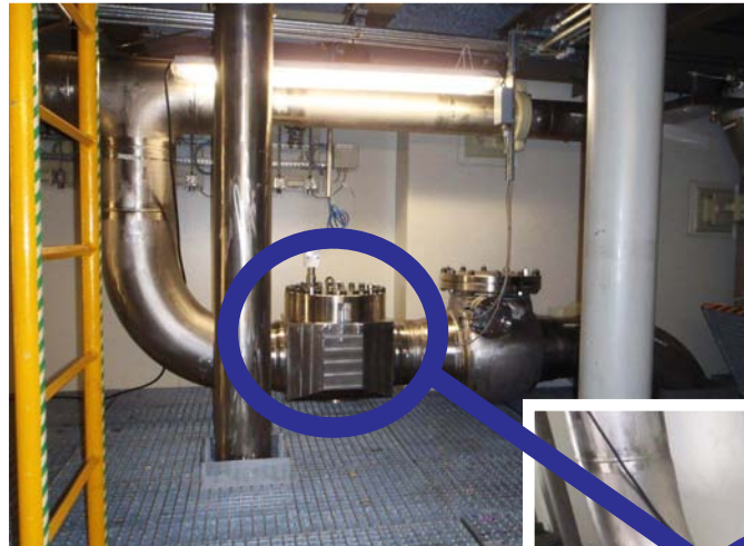
Fig. 1: The new second check valve.
