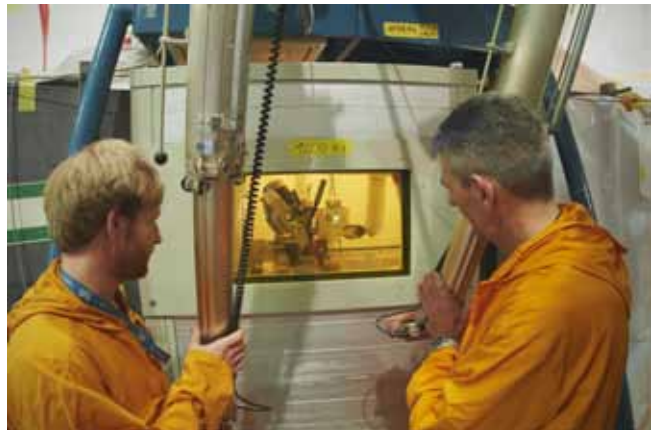
Fig. 3: Michael Schulz (l.) and a contractor working at the temporary hot cell in the experimental hall to dismantle parts of the beam tube SR11.
