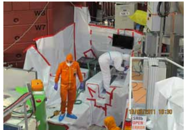
Fig. 4: Construction work at the HEiDi site during the reactor shutdown in March 2011.
