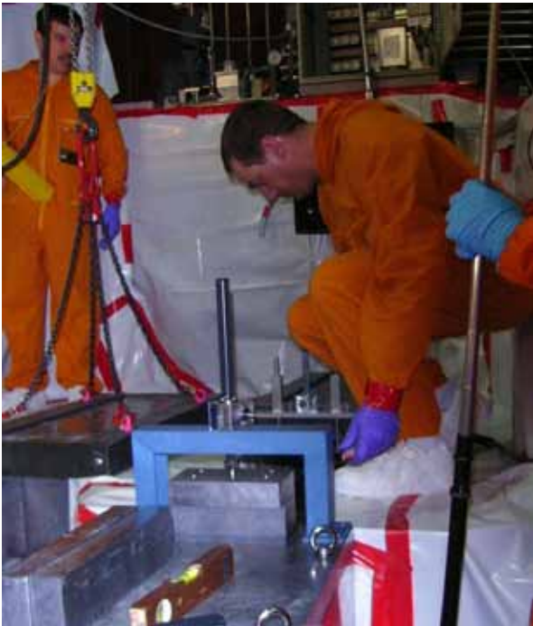
Fig. 2: Works at the beam tube pointing at the hot source to feed the new instrument POLI@HEiDi with hot neutrons.
